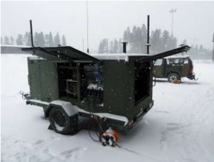
1521991 - Powered up view of the M18 Communications Trailer E module. Visible here are the Band I antenna, Multiplexing, CNR and EB Radio Head I Unit (Band I). (IHS/Konstantinos Tigkos)
