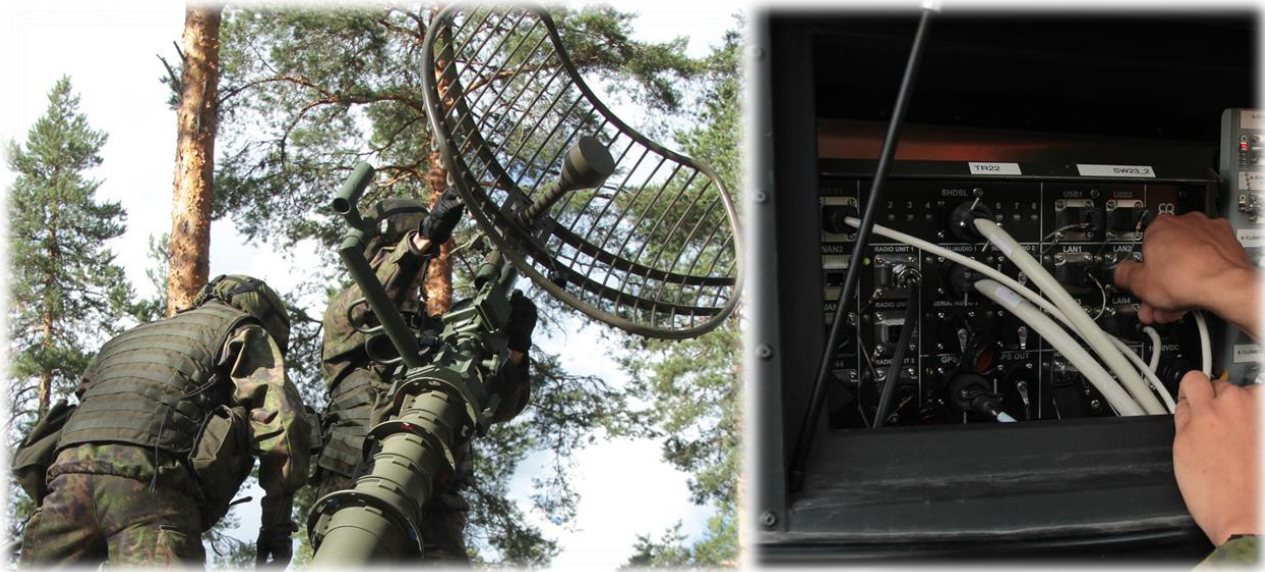
EB Tactical Wireless IP Network (TAC WIN) installed in an army vehicle. Copyright Finnish Defence Forces
